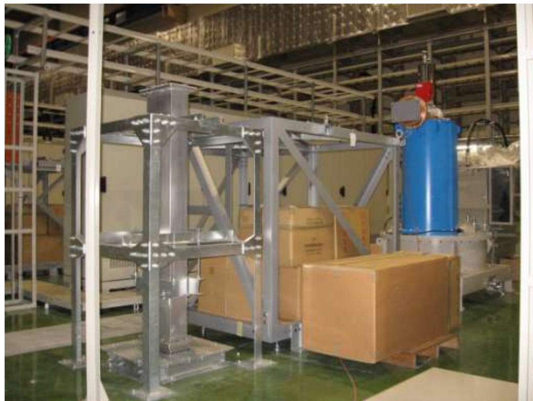
Waveguides were installed from the klystron gallery to the accelerator tunnel during the summer shutdown in 2009.
