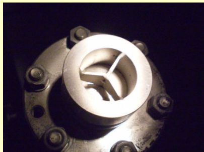
Q8R3 V1: rupture disk deformed but not perforated
