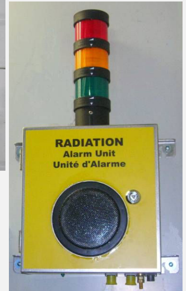
Radiation Alarm Unit (RAMSES)
