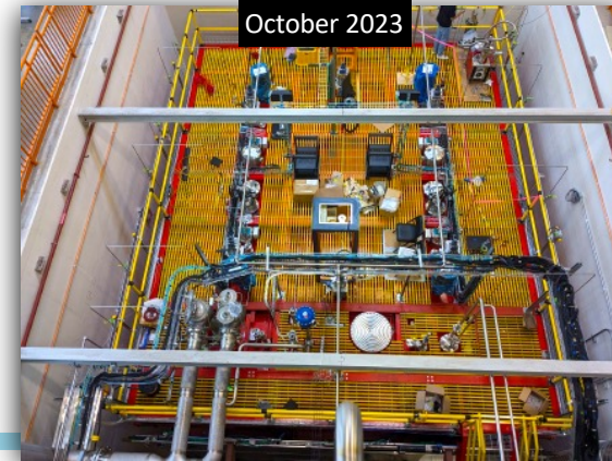
Cabling and cryogenic connections
