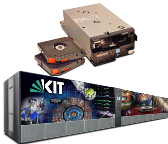
top: tape cartridge & drive, bottom: tape library at KIT (current total capacity: 150 PB)
